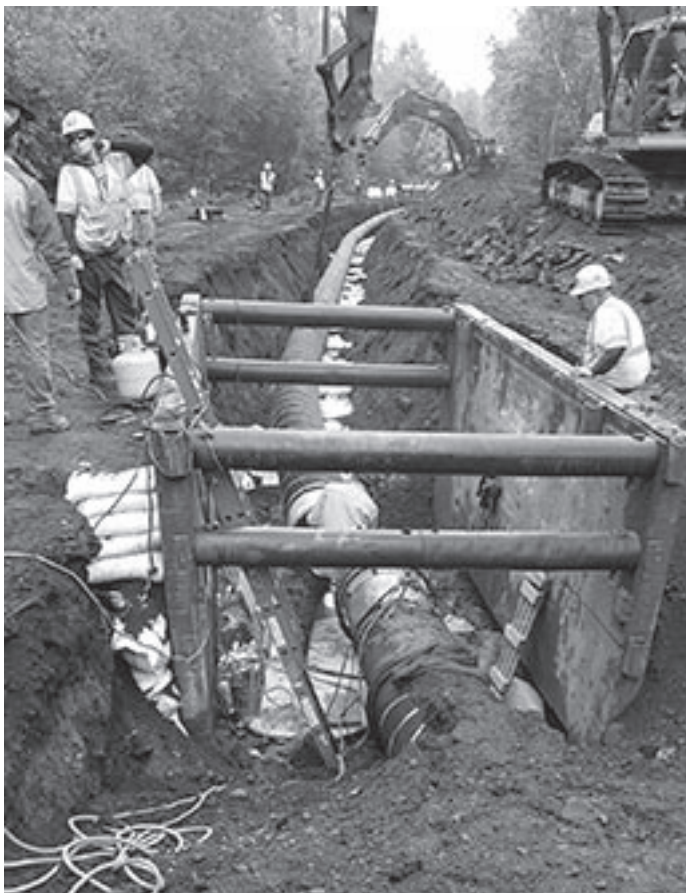
It took 18 workers about 45 minutes to gently guide this curved 500 foot section of 36 inch steel pipe into a position to attached it to an already installed underground pipe. A worker on a walkie-talkie relayed instructions to each of the four excavator operators to make movements of fractions of inches to align the pipes for welding.
