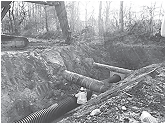
Pictured is a drainage cross pipe under the 16" and 24" natural gas pipelines on the D&H Rail Trail.
